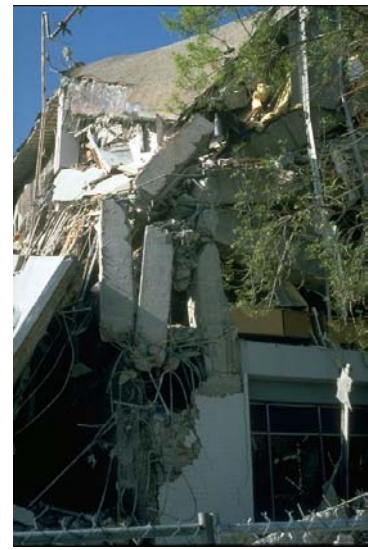
Figure 4 – Joint failures – Northridge earthquake
