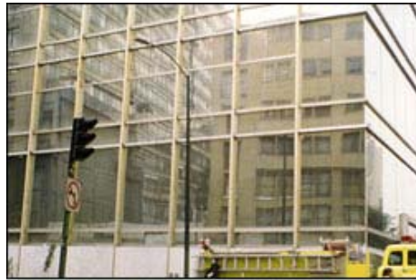
Figure 3. Only minor glass damage occurred to this bank in downtown Mexico City, in one of the areas most severely shaken in the earthquake of 1985. Note the undamaged mitered glass at the corner.
