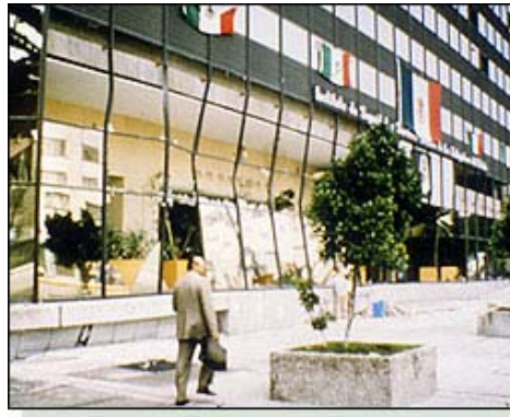
Figure 19: Glass damage in Mexico City earthquake, 1985. Note the extreme distortion of the first floor, but only a few glass panels were severely damaged. Even with the massive shaking, glass in the upper floors is undamaged.
