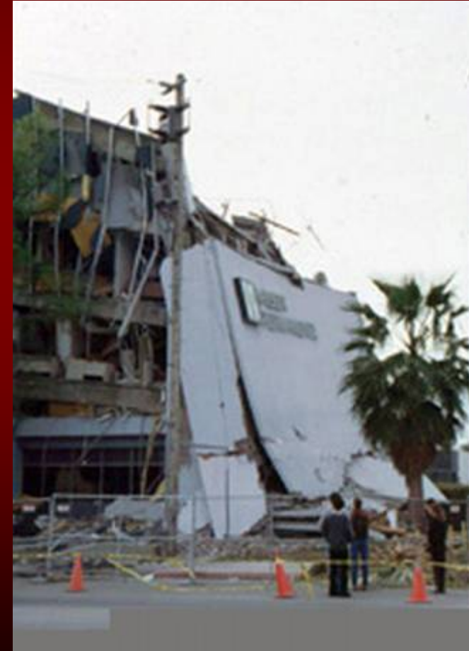
Collapsed side wall
