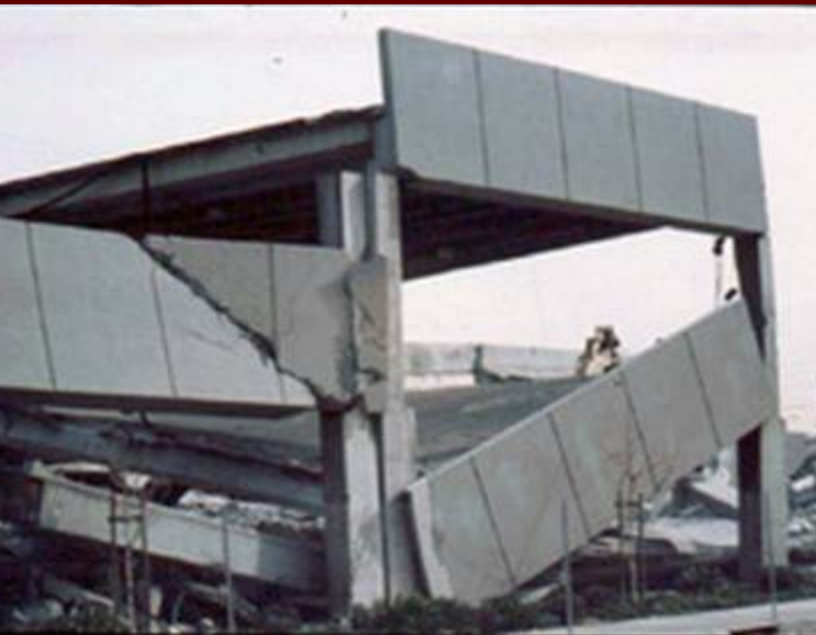
Prefab parking garage parapet failure
