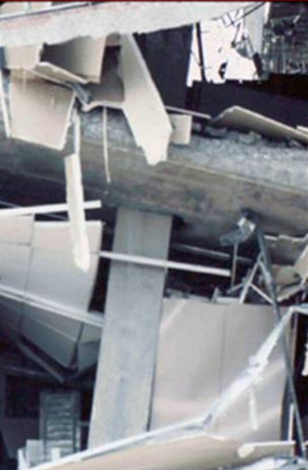
Column punctures concrete slab
